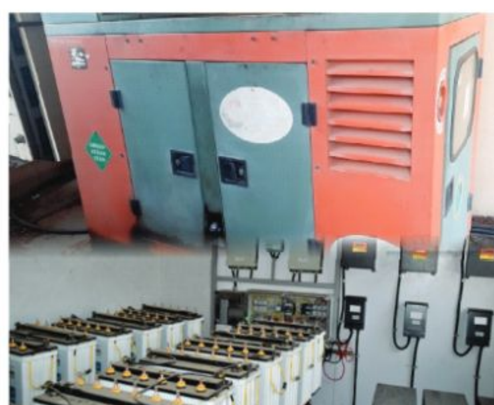
Power Generator and UPS Back-up
